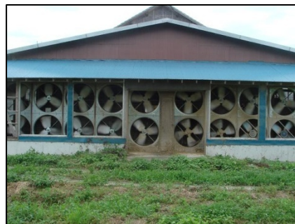
↑牛舎壁面の換気扇
